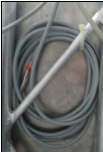
Figure 18: Not connected Pyrriadiometer cable
